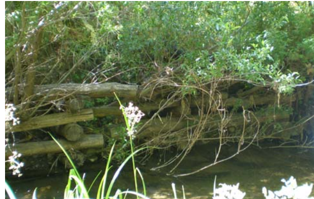
A bio-engineered crib wall was installed to stabilize Palomares Creek. This WHIP project launched several other community-based watershed improvement activities.
